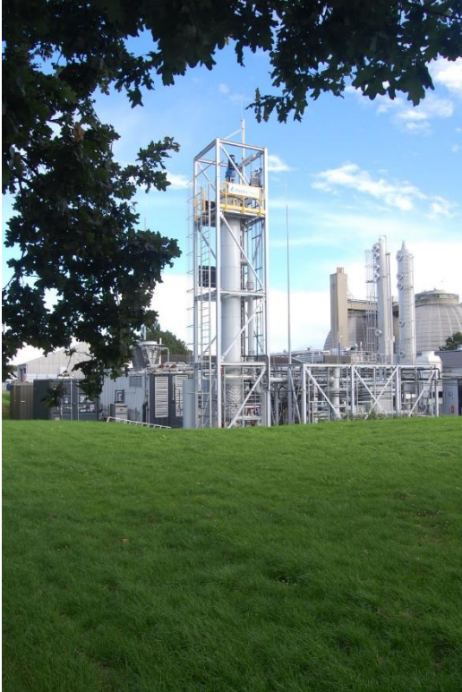
BioCat Pilot Plant Denmark ©Electrochaea GmbH
