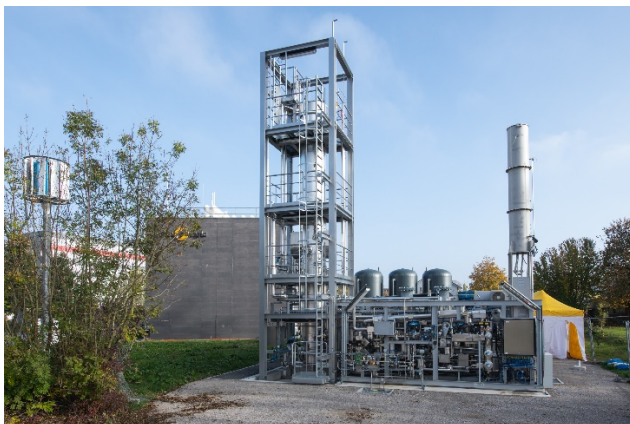
The power-to-methane plant, a joint project between Electrochaea and Regio Energie Solothurn. Here, excess electricity and biogenic CO 2 are converted into renewable methane for the Swiss gas grid. (c) RES, 2019.
